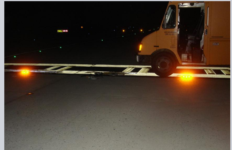
L-852G LED Test Installation at Atlanta- June 2008
